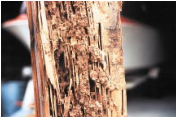
Fig. 7b. Subterranean termite damage.
