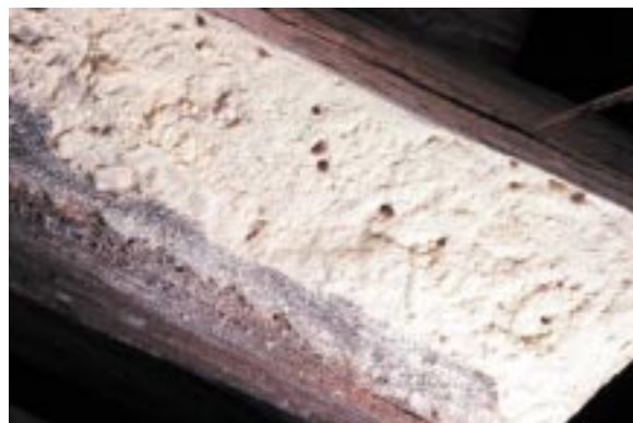
Fig. 4d. Lyctid beetle damage.
