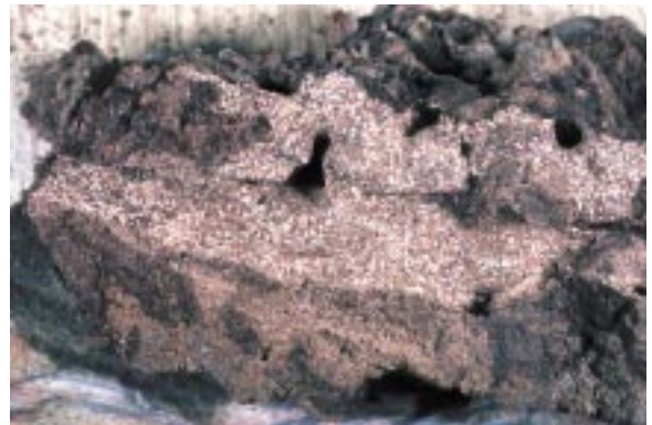
Fig. 7a. Subterranean termite "scaling."
