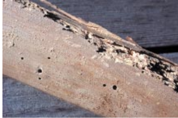
Fig. 3. Shot holes in wood. (Lyctid or powderpost beetle exit holes.)
